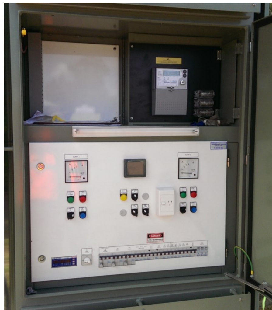
SPS - Pump Control Instrument Panel
