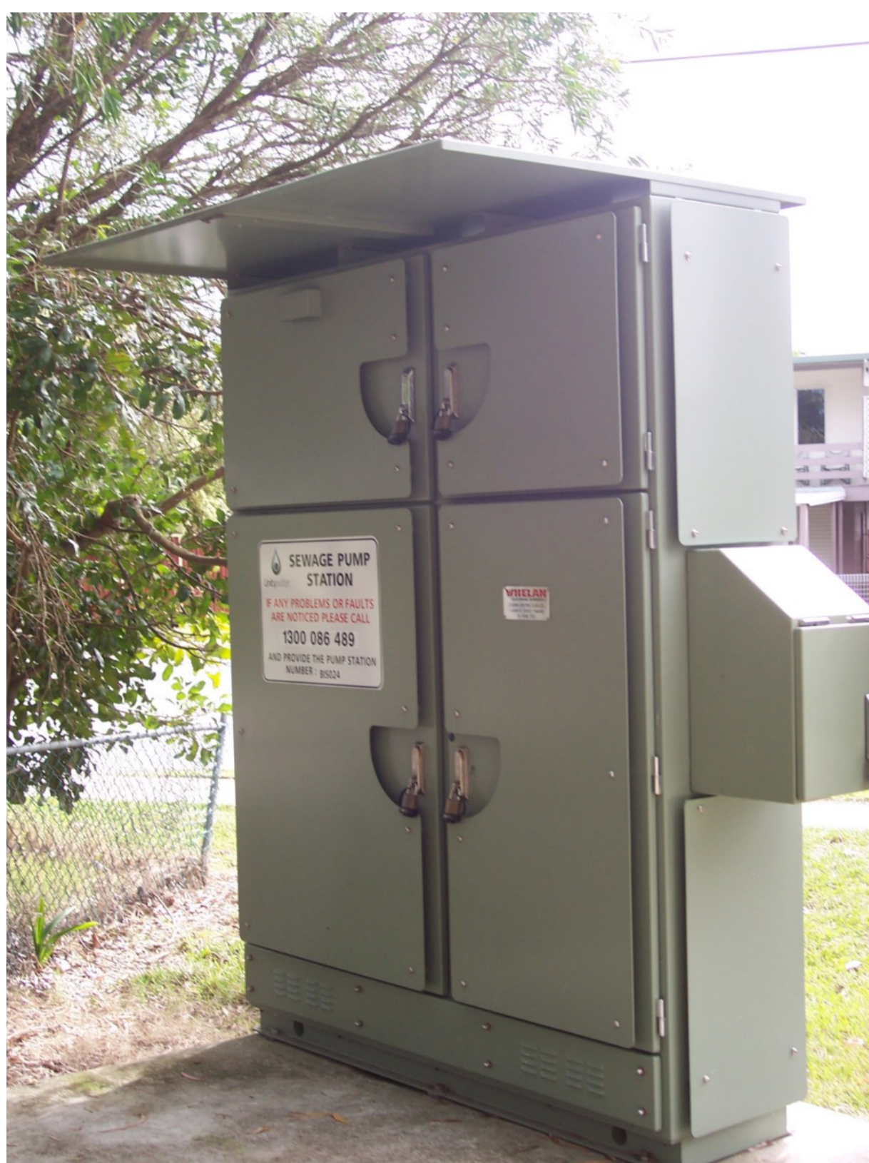
Example of one of Unitywater's Sewage Pump Stations
