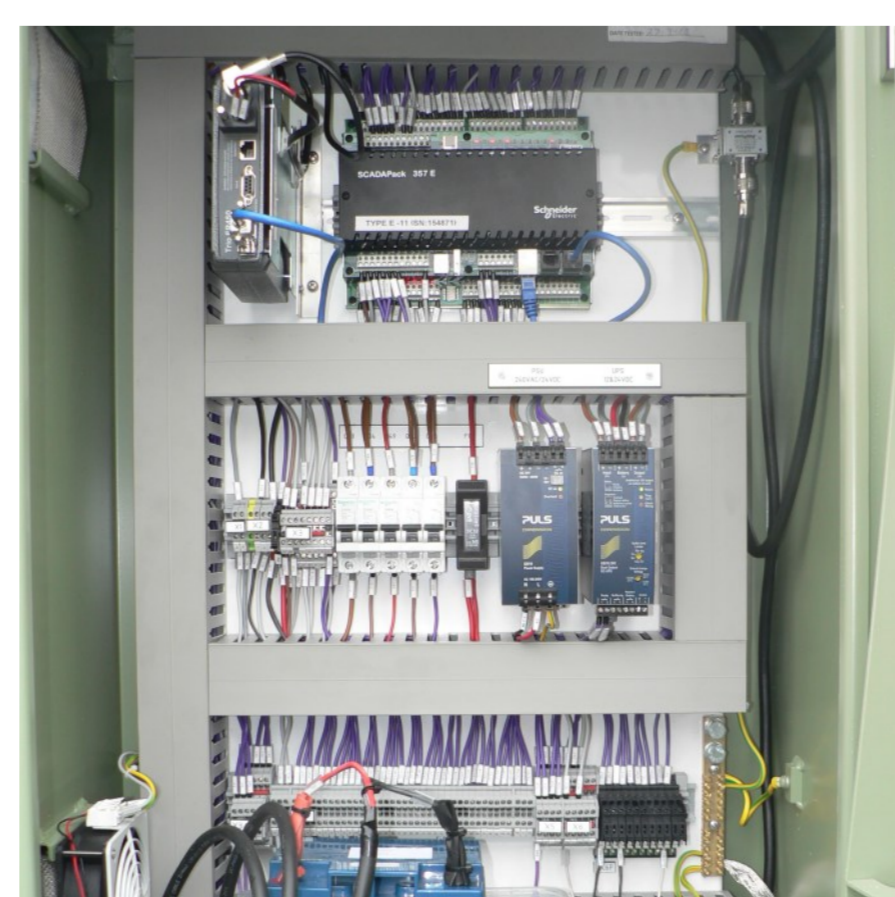
SPS - SCADApack RTU Section
